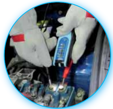
Voltage detection on electrical power circuit.
